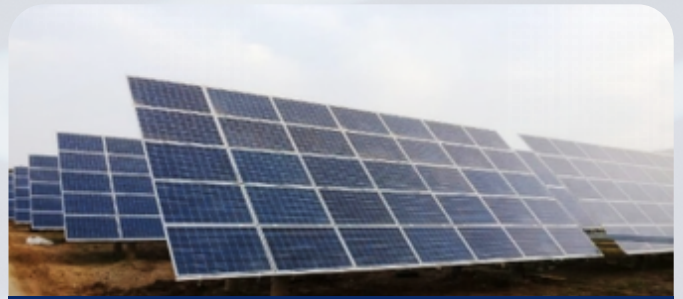
C & I, Telangana, 2.50 MWp Single Axis Tracker
