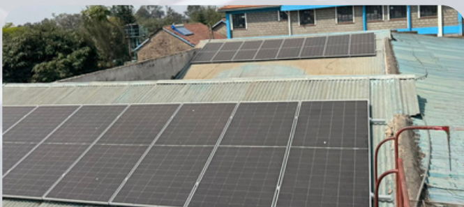
EPC, Kenya, 61.38 KWp
